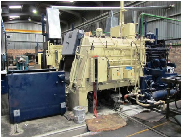
Today the company's facilities include six Ipsen and four Efco and Birlec sealed quench furnaces using Afrox's Endomix system among its extensive range of capital equipment
